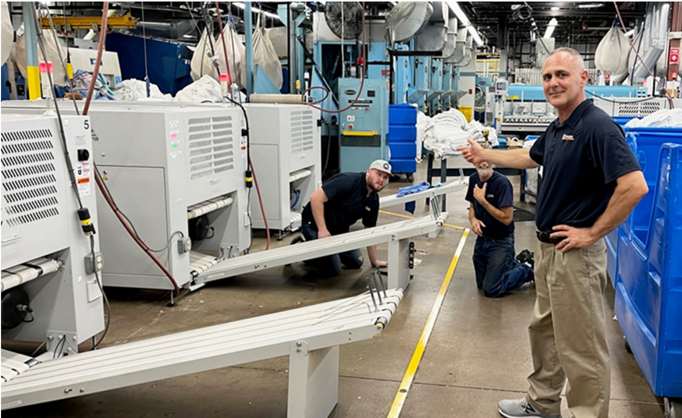
Regional Manager for New England, Ray Neal , supervised the placement and installation. By the next day, the new Foltex machines were pumping out linen!
